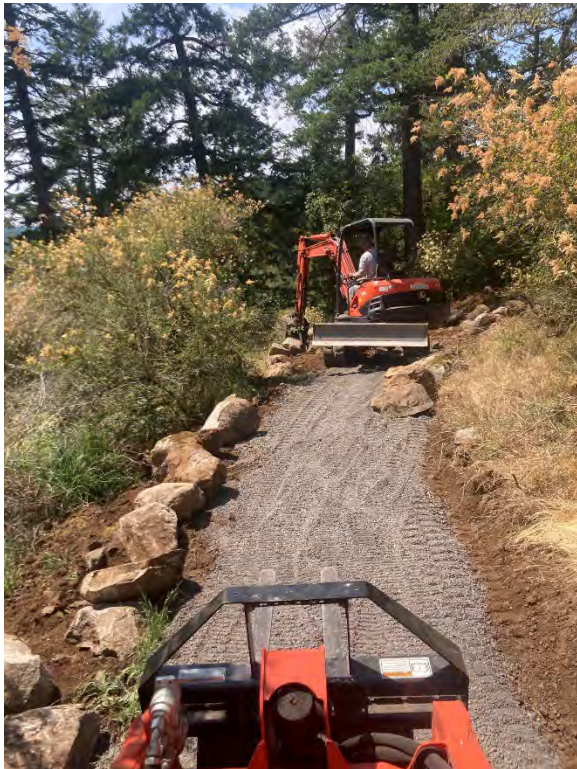
Photo 4. View from Kuby (our mini track loader) of EcoEarthworks building rock retaining wall at Beaverton Marsh Viewpoint
