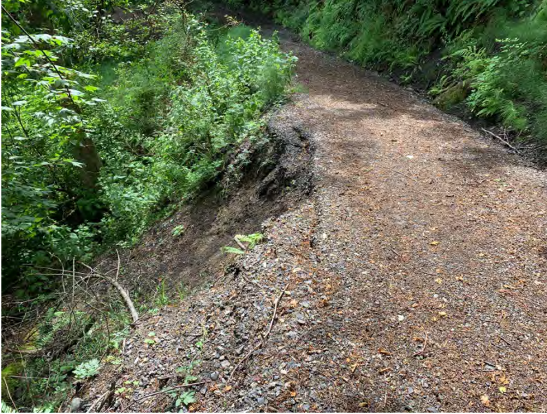
Photo 3. Slope failure requiring attention along the beach access road at the North Shore-Glenwood property.
