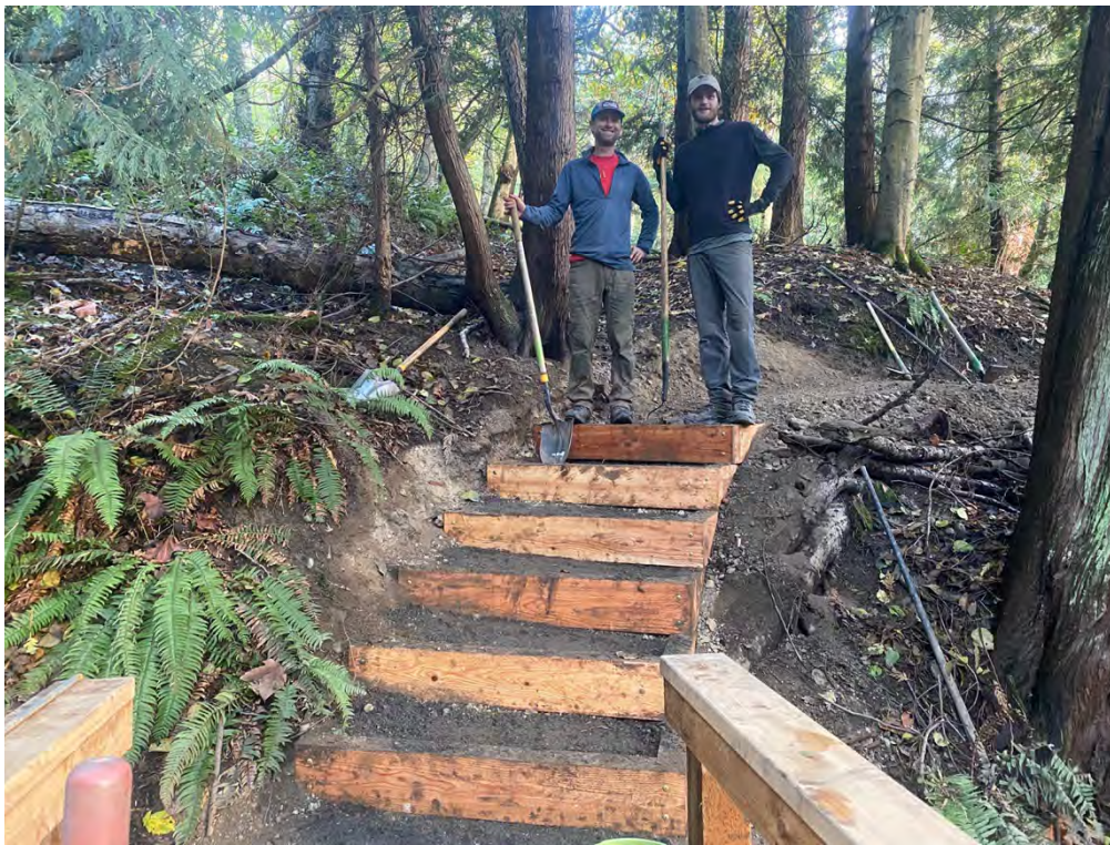
Photo 5: Andrew and Jacob stand proud on cedar box steps installed at Turtleback.
