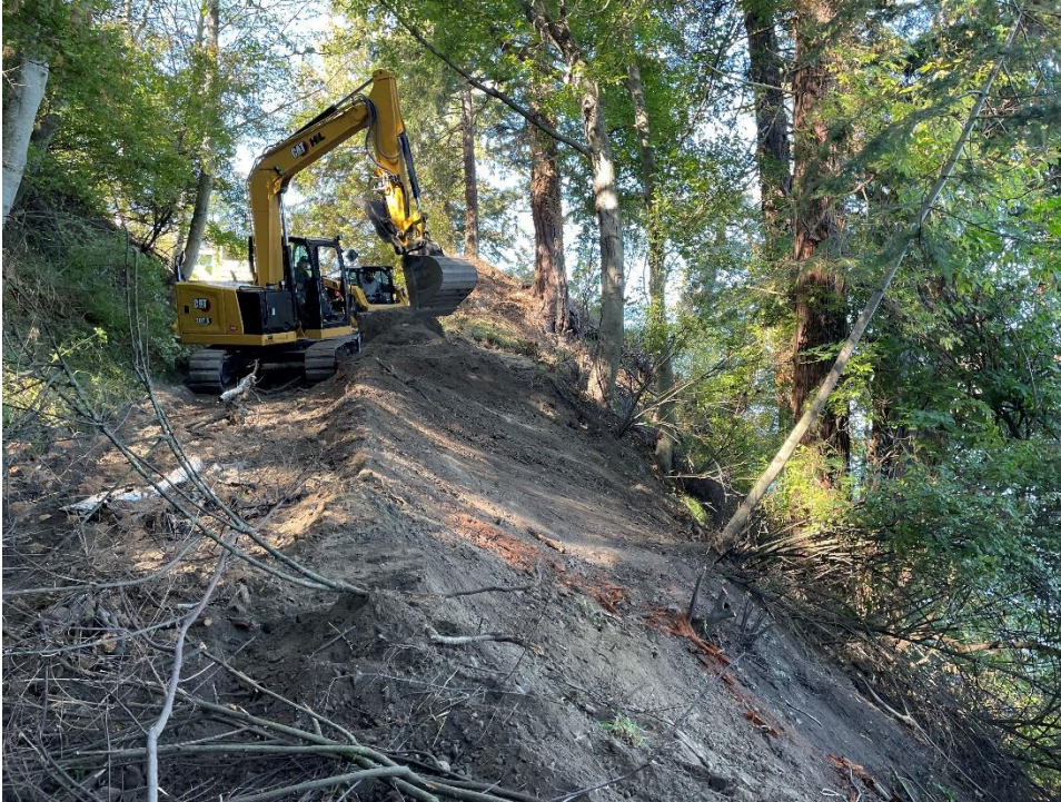
Photo 12. Preliminary grading of the old road to remove slide material, North Shore Preserve.
