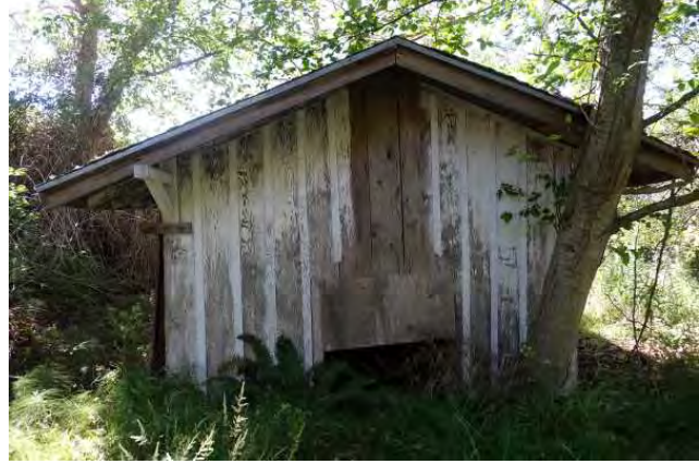
East side of cottage, showing former location of chimney; view to the west.
