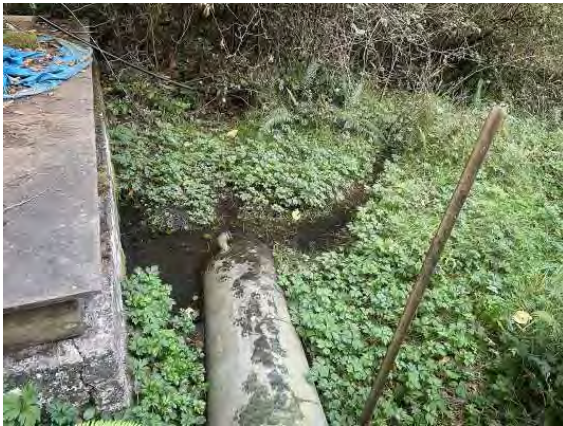
Water flowing behind spring box; abandoned equipment in foreground; view to the southwest.
