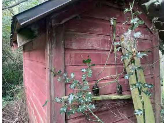
Back of pump house, showing electric components; view to the west.
