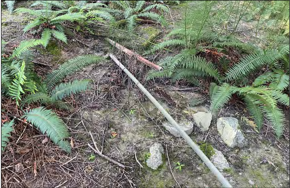
Figure 36: View northwest, pipes protruding from hillside.
