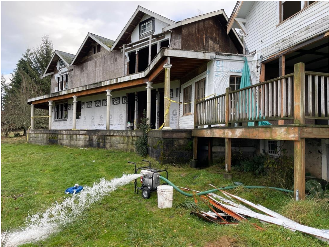
Photo 3. Pumping out the basement and preparing for an asbestos inspection at North Shore Preserve.
