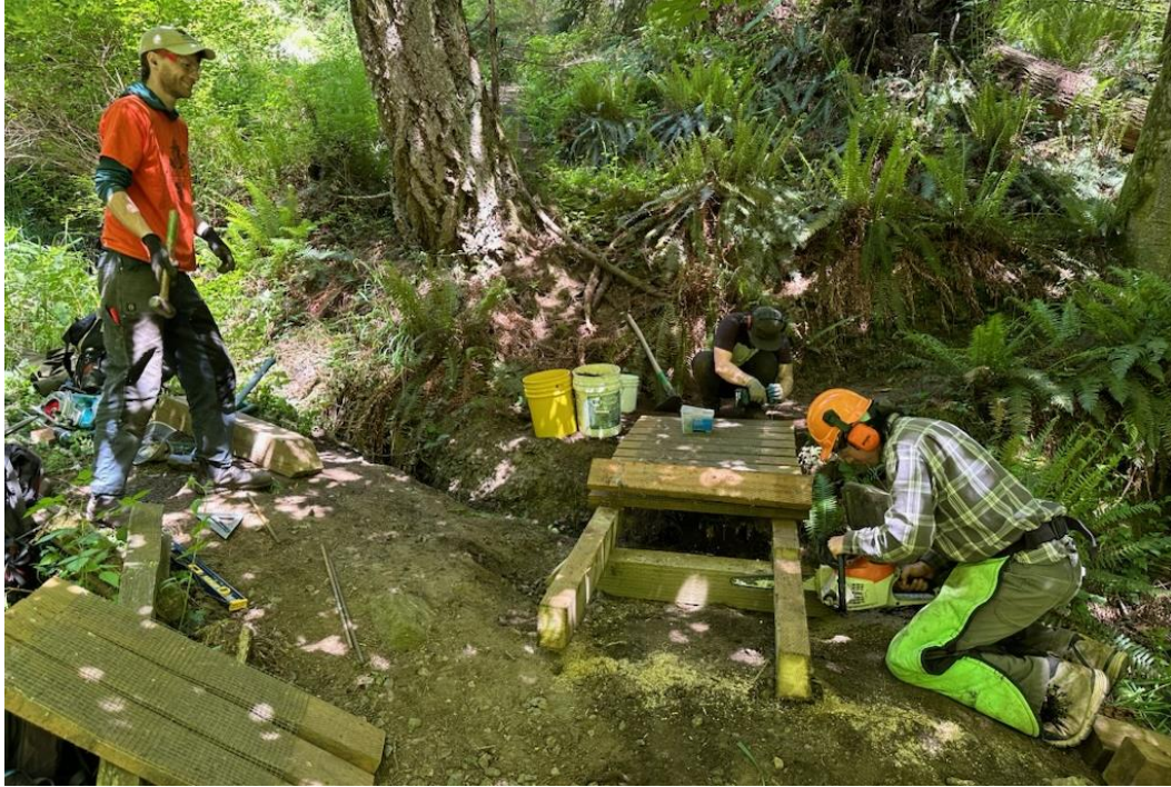
Photo 16: ICC members work on repositioning a pre-existing bridge to flow better with trail movement, Coho Preserve.
