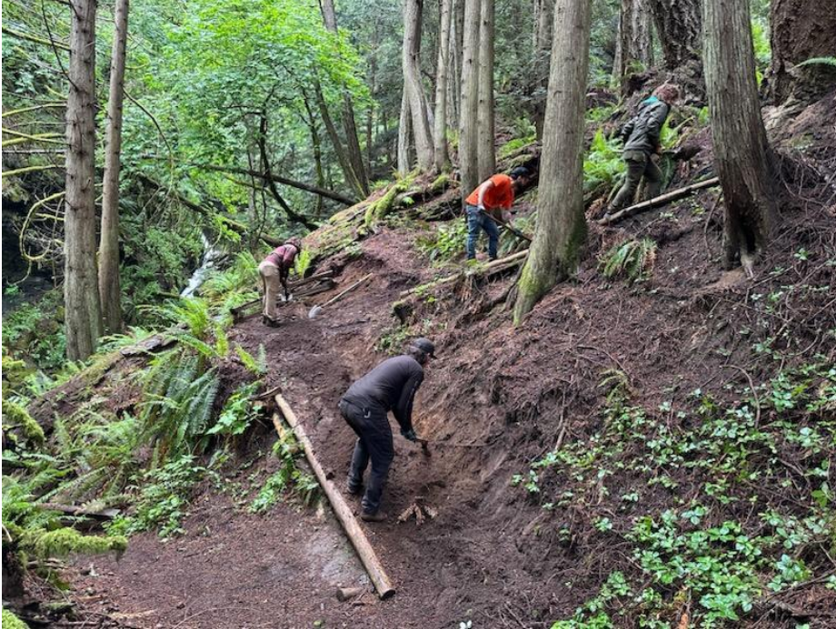
Photo 2: ICC members work on widening switchbacks and re-building retaining walls, Coho Preserve.
