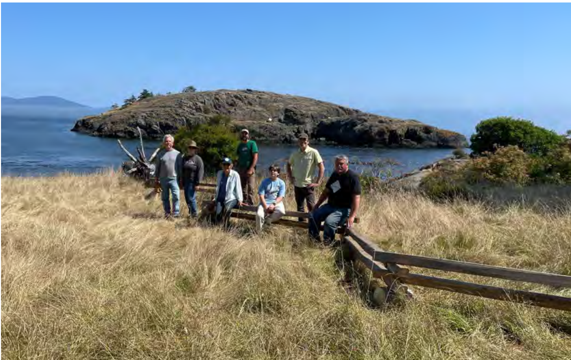
Photo 19. Volunteers help construct a split rail fence on the headland at Watmough Preserve
