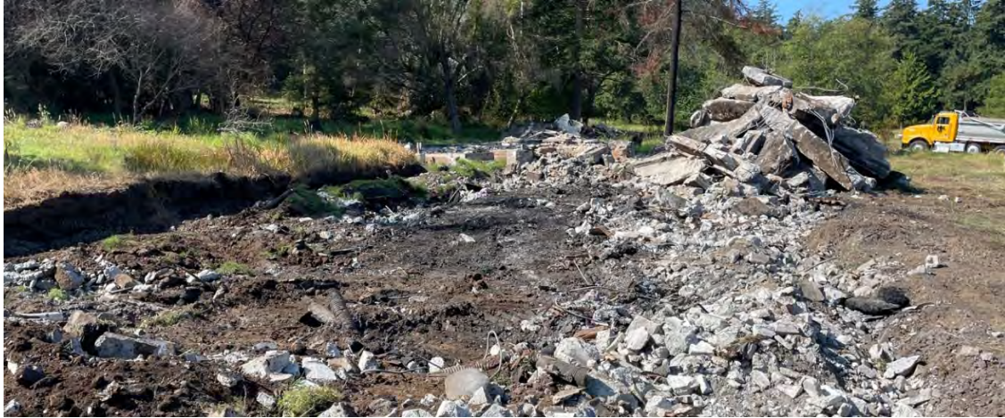
Photo 12. The foundation of the old house was demolished and hauled away, at North Shore.
