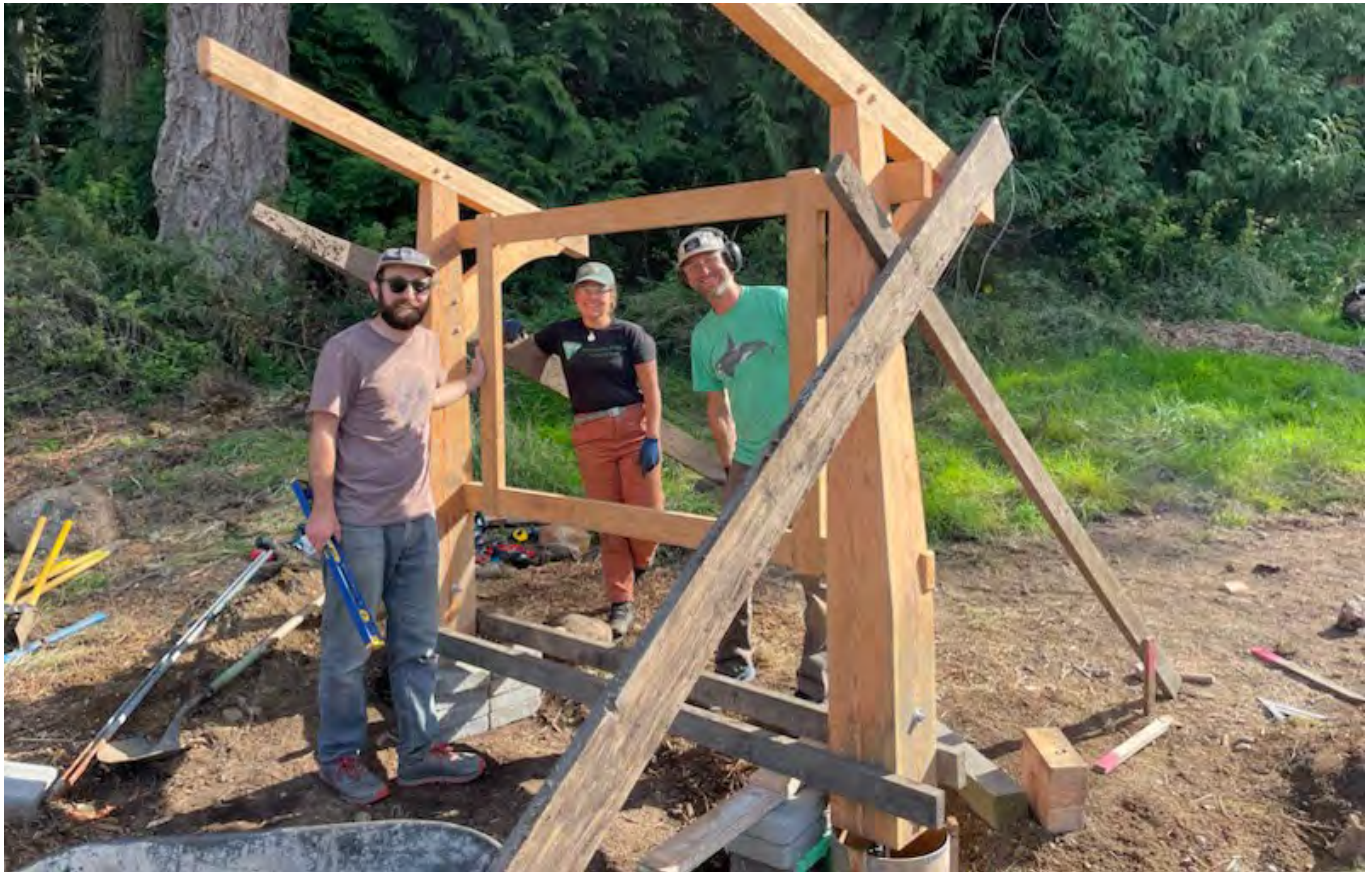
Photo 5: Tyler, Shauna, and Jacob install the volunteer-built kiosk at North Shore Preserve
