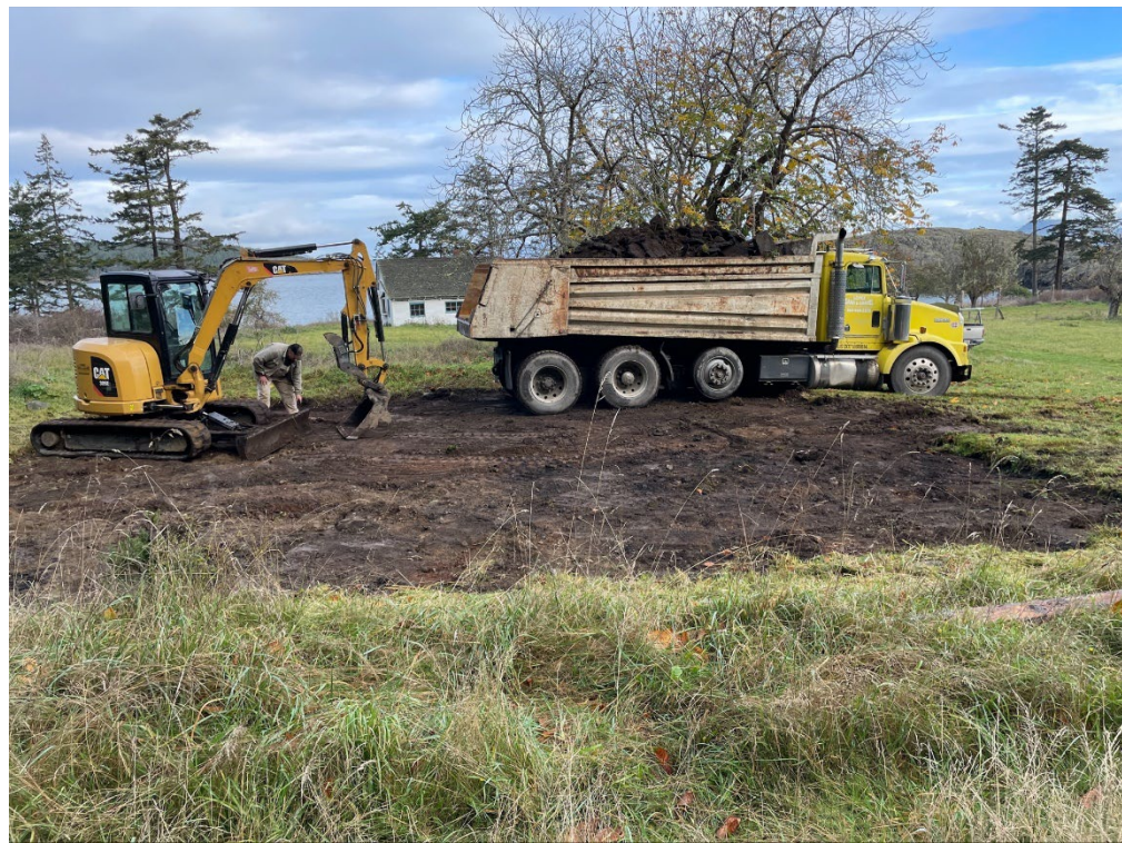
Photo 10. An asphalt pad was removed from the headland at Watmough Bay Preserve.
