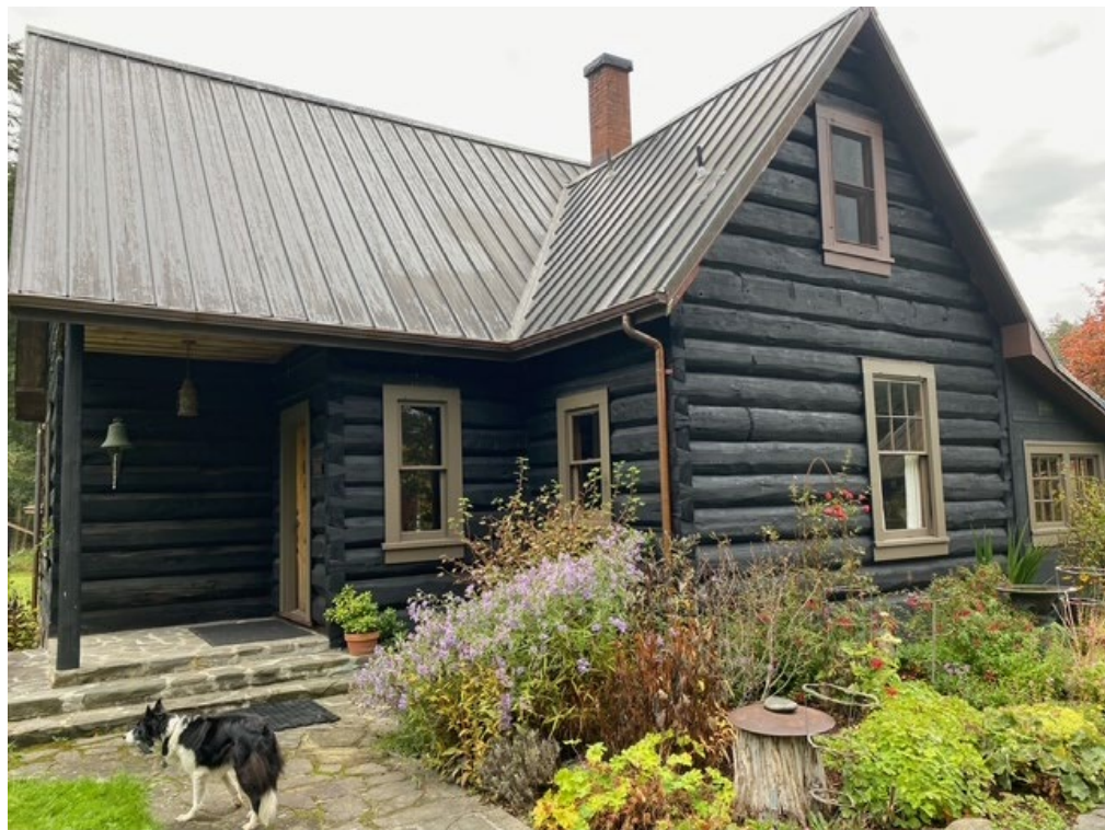
Photo 8. SJPT's Tharald Homestead, protected by a conservation easement, was outfitted with new gutters and downspouts, Shaw Island.
