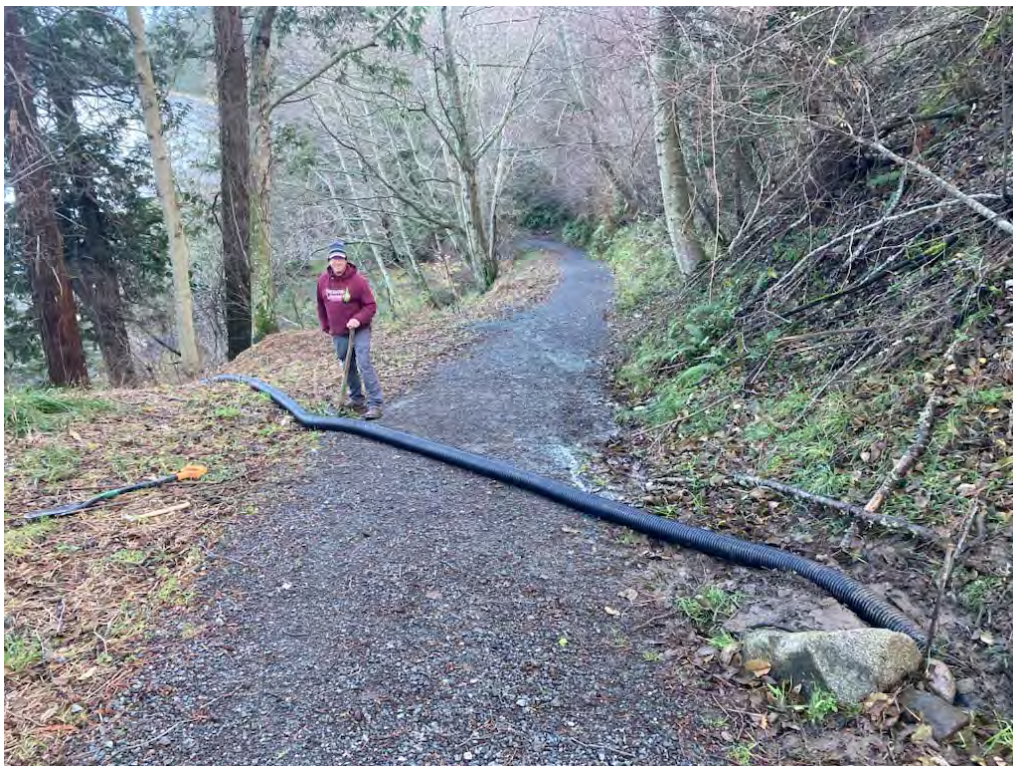
Photo 6. Volunteer Jonathan Heverly assisting with North Shore 'emergency' drainage diversion following atmospheric river.
