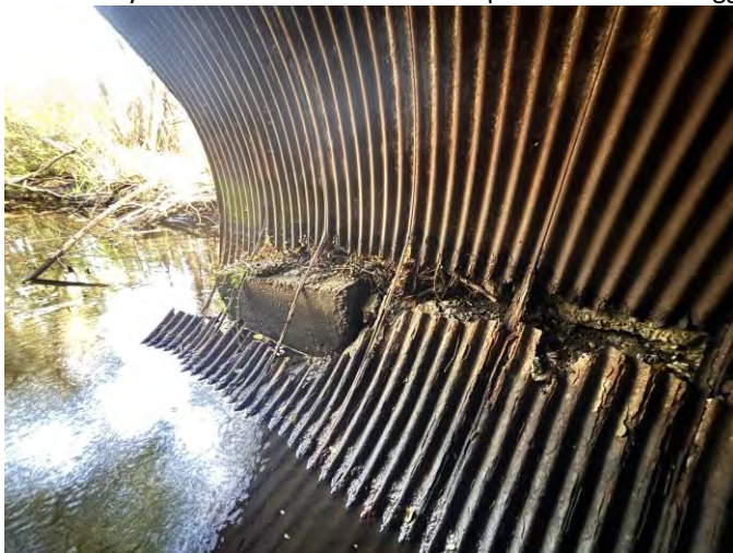
Photo 9. Failing culvert at Zylstra Lake Preserve.
